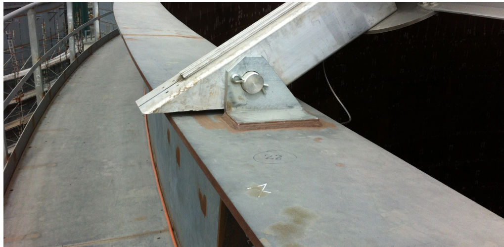
Fiber optic sensor cable mounted around the tension ring at the top of the tank, and along the outside wall
