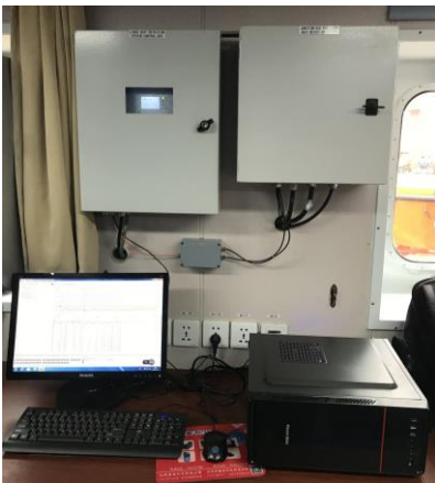
DTS installed in control room
