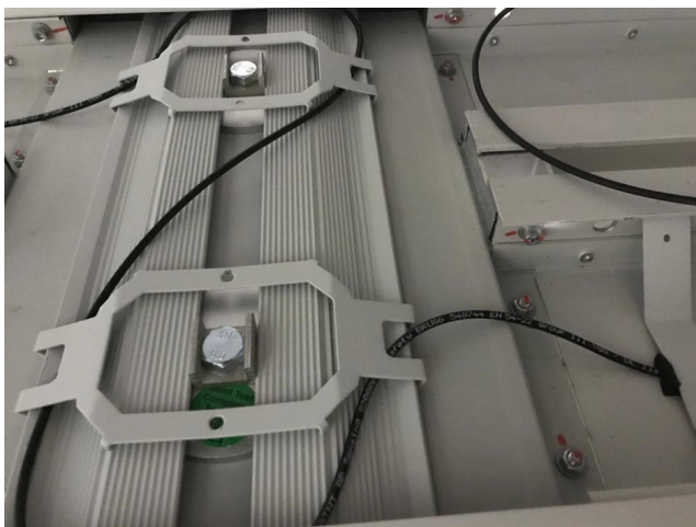
Sensor Cable on E&I 3200A Bus Duct Joint
