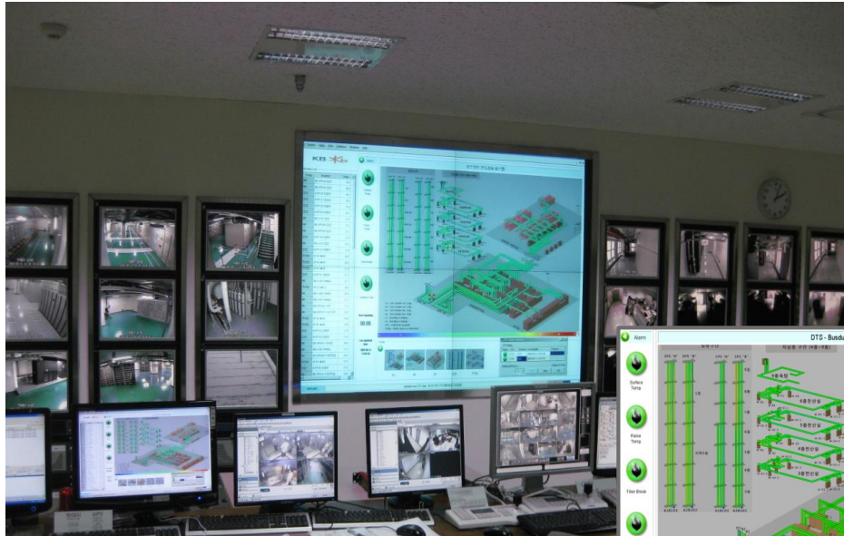
Central Control Room
