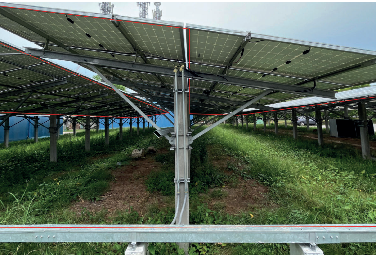
Figure 2: Greenfield solar installation with AP Sensing's fiber optic LHD system shown in red for visibility, running underneath the panels.
