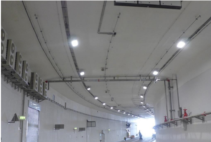
The Saadiyat tunnel with sensor fibers installed
