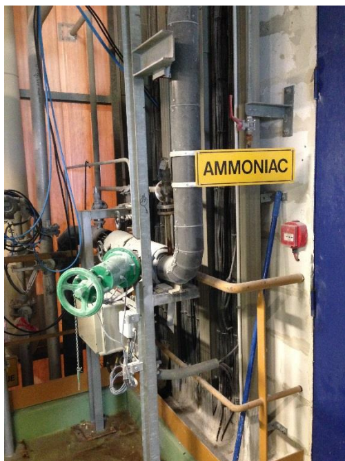
Ammonia pipeline area
