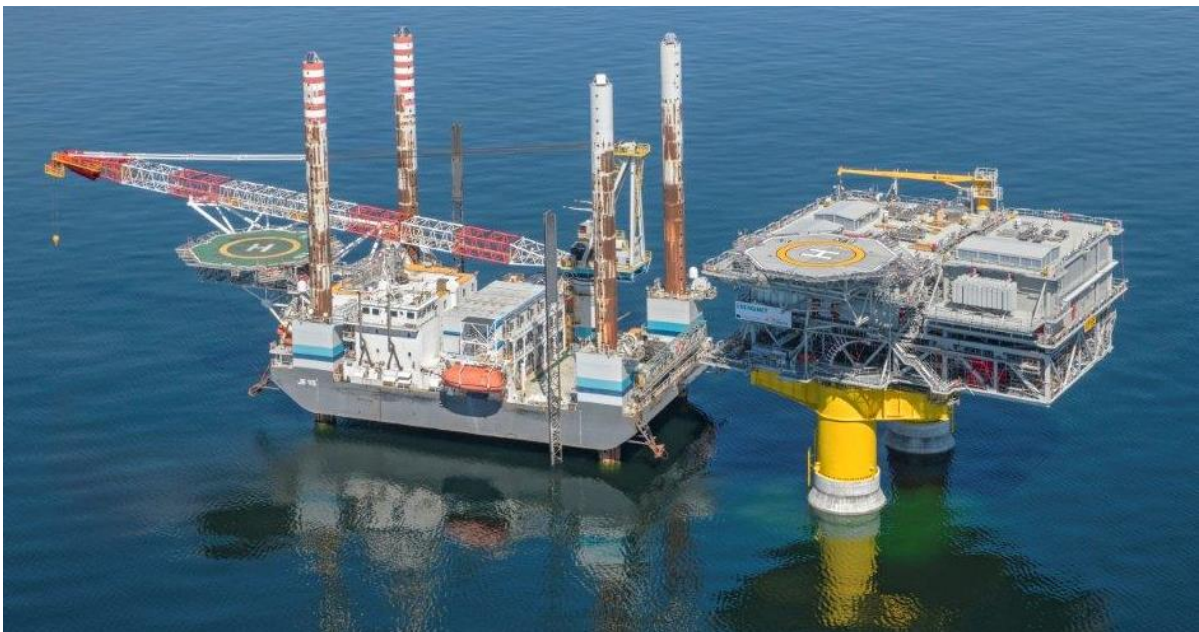
Kriegers Flak offshore wind farm ©Energinet
