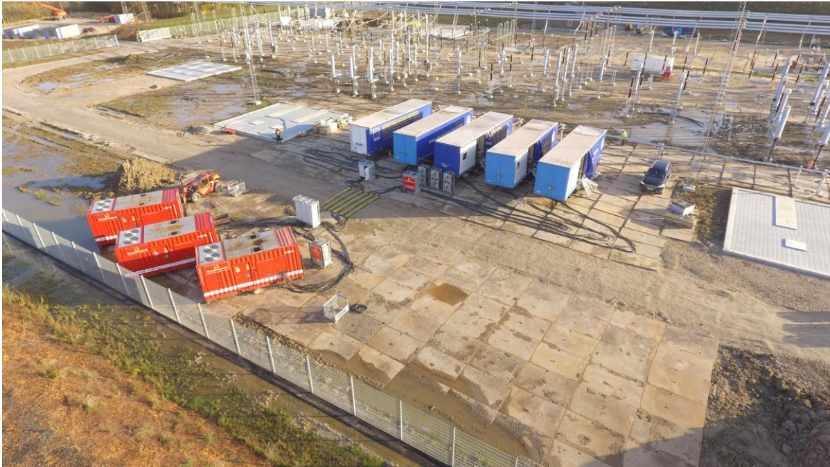
Bjaeverskov substation setup ©Energinet
