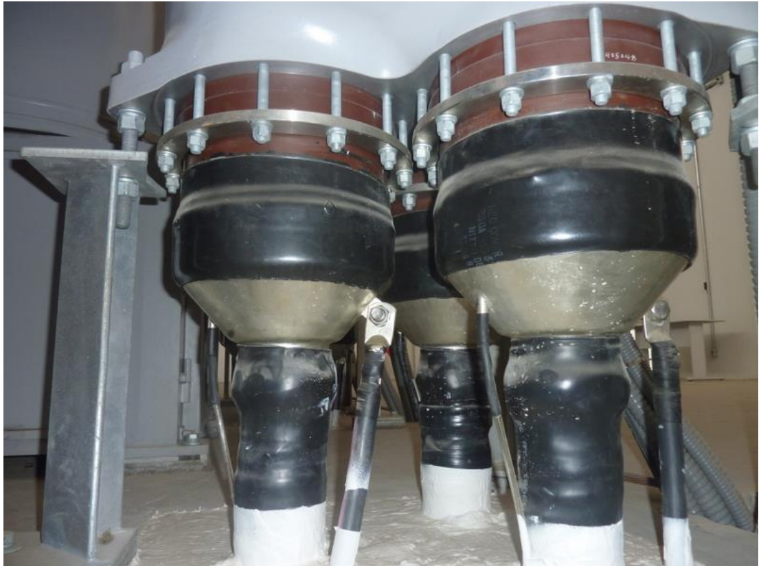
GIS termination showing the 3 phases
