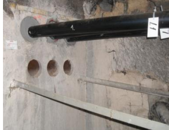
Cable enters the utility tunnel
