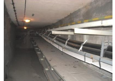
Cable in utility tunnel
