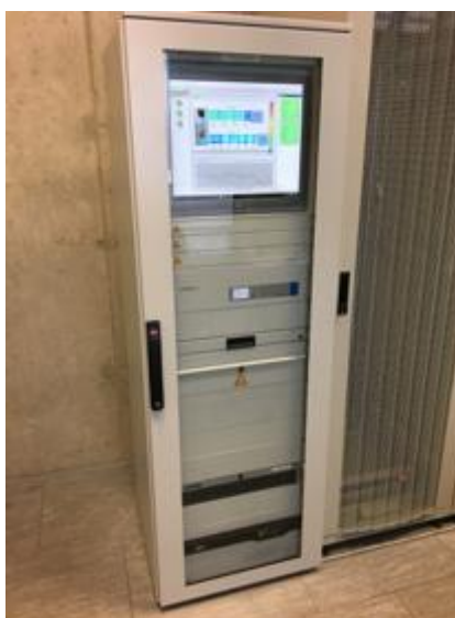
Operation of a DTS unit in a rack
