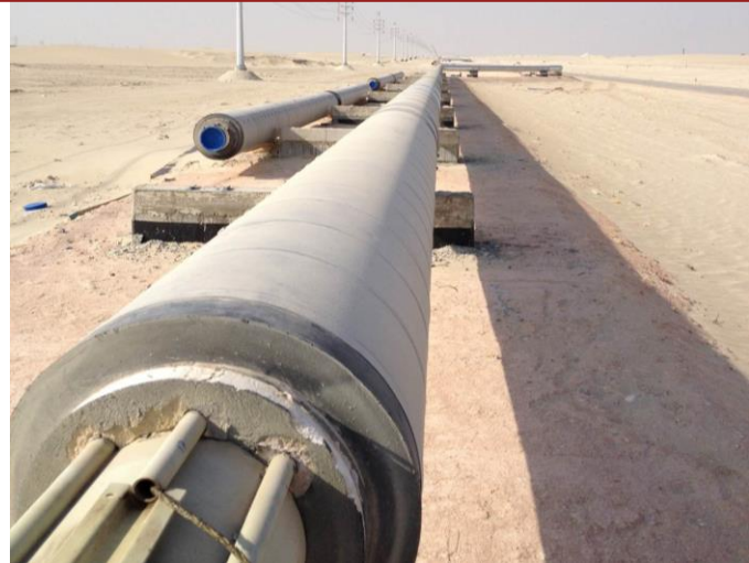
Sulfur pipeline utilizing AP Sensing monitoring solution
