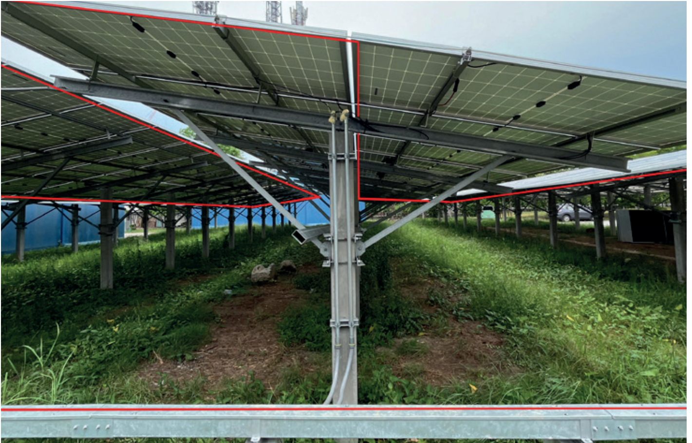
Greenfield solar installation with AP Sensing's fiber optic LHD system, shown in red for visibility, running underneath the panels.
