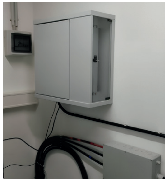
19" AP Sensing DTS device mounted in a flat wall cabinet
