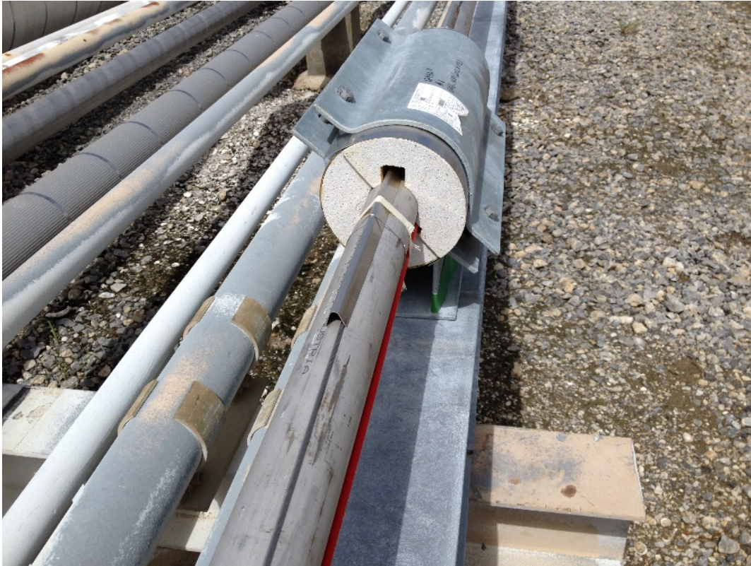
Phenol transport pipelines with heat tracing
