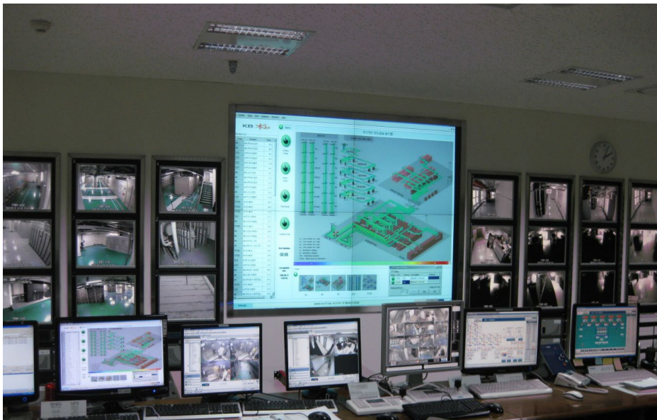
Central Control Room and 3D Asset Visualization
