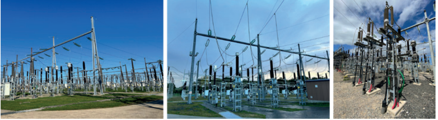
Figure 1: Power cable terminations in the substations of (left) Fécamp, (middle) Saint-Brieuc, and (right) Gruissan offshore wind farm projects.
