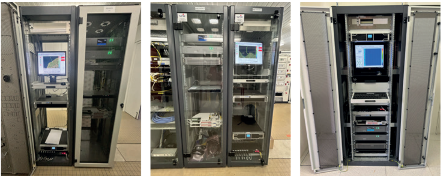
Figure 2: Monitoring racks in the substations of (left) Fécamp, (middle) Saint-Brieuc, and (right) Gruissan offshore wind farm projects.
