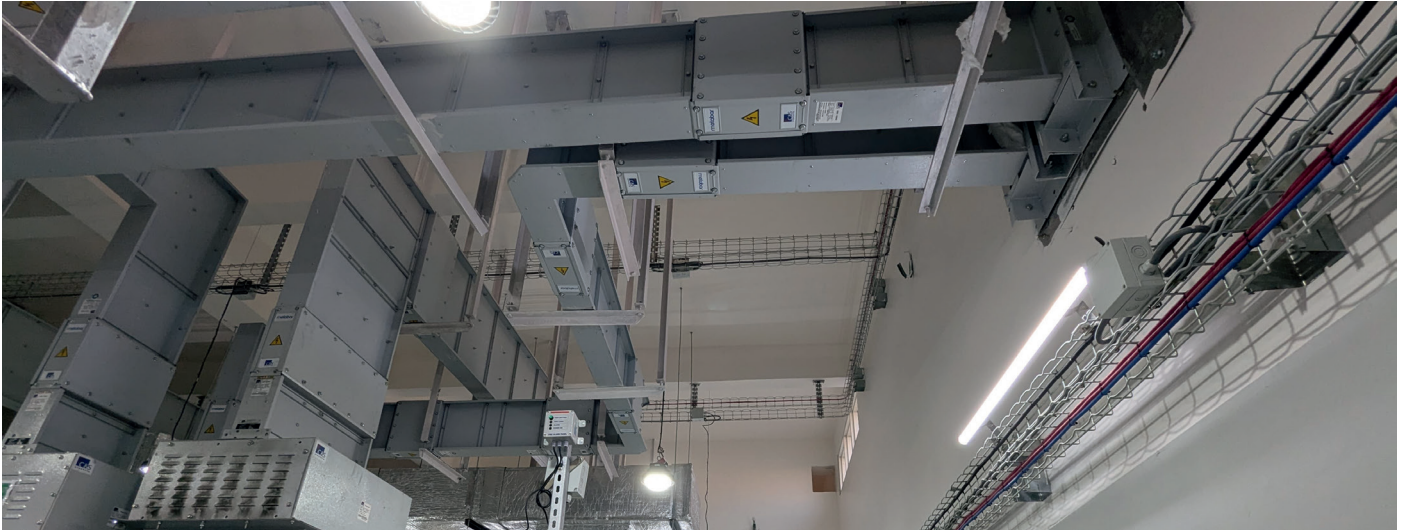
Figure 1: Bus Ducts at Nestlé Plant in Sanand, Gujarat, India
