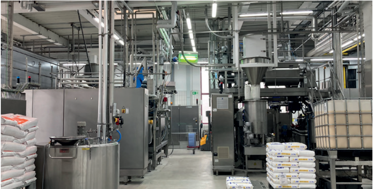
Figure 1: Production areas, machinery and equipment create a complex environment. Reliable fire detection must provide comprehensive coverage.
