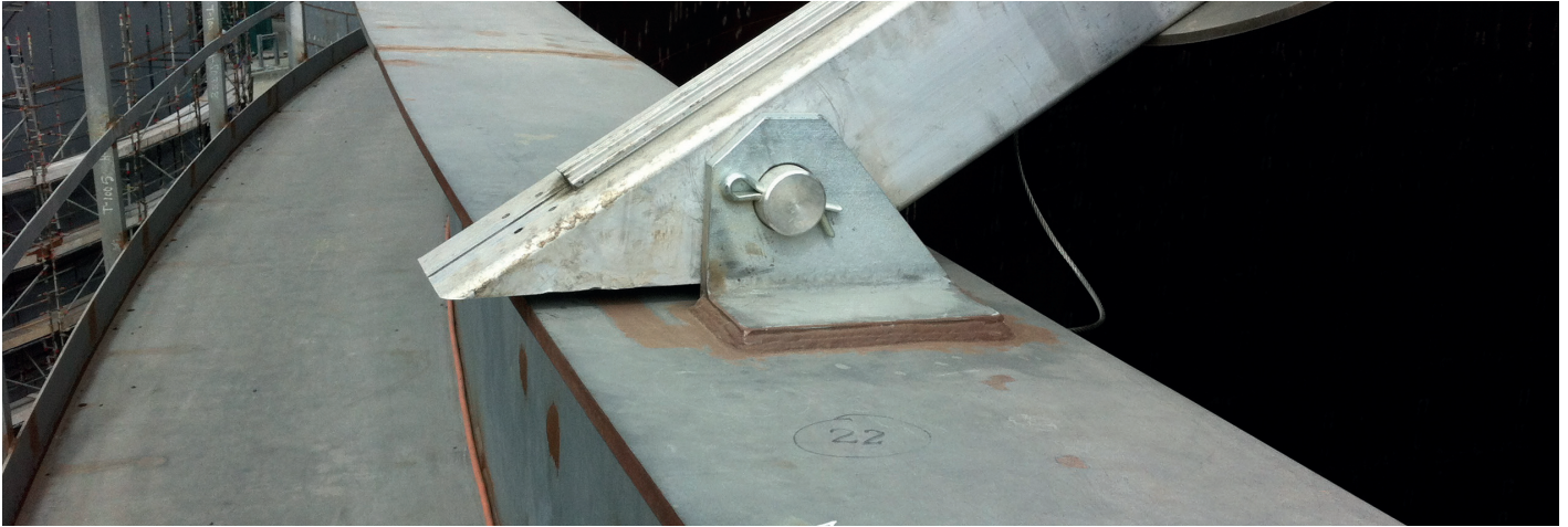
Figure 1: Fiber optic sensor cable mounted around the tension ring at the top of the tank, and along the outside wall
