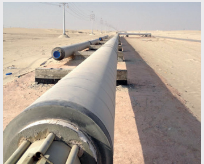
Sulfur pipeline utilizing AP Sensing monitoring solution
